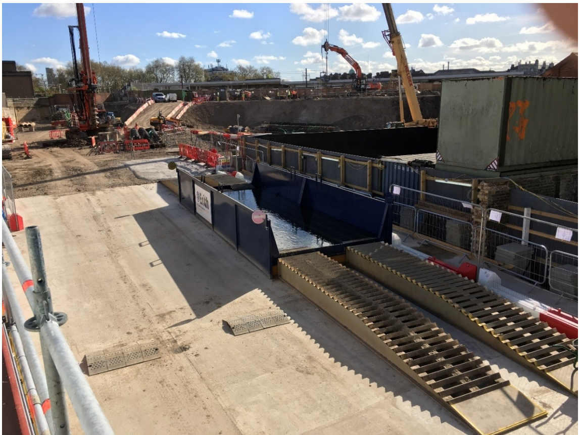
Figure 1: Example of a drive through wheel washing facility
